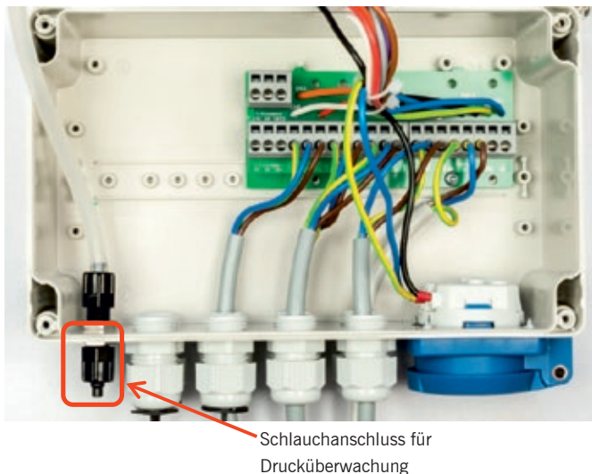
Figure 5: Hose connection for pressure monitoring
